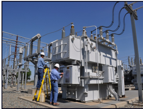
MID workers perform maintenance on one of the District's many transformers. MID is trying to minimize energy costs from a state mandate.
